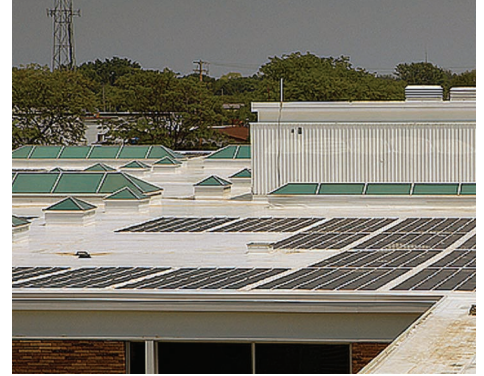
More than 14,000 square feet of thin-film PV cells are laminated to the roofing membrane of one building to generate electricity.
