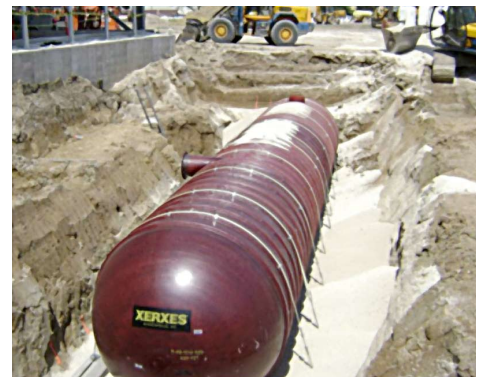
By capturing rainwater and snowmelt in this cistern, then cleaning and reusing it, municipal water use is reduced by 77 percent.
